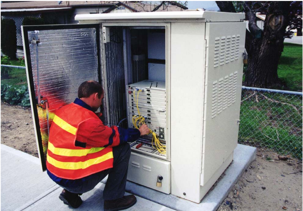
The Douglas County Community Network (DCCN) connects Douglas PUD's substations, administrative offices and Wells Dam to enhance the efficiency and safety of the electric system.
